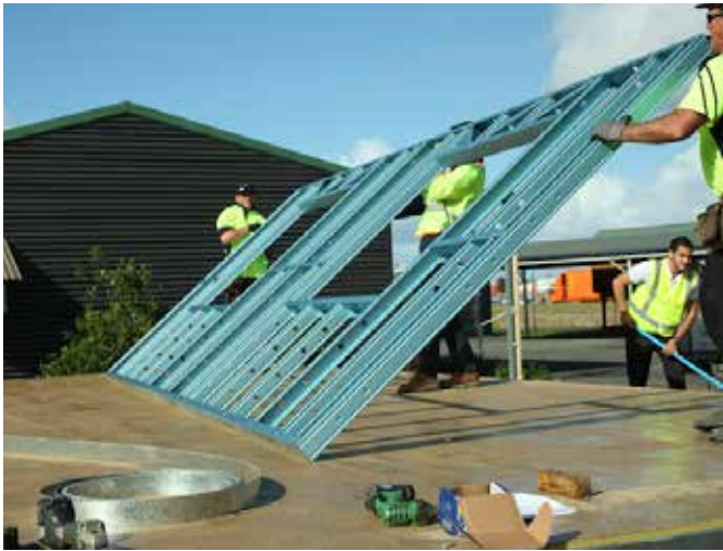
Figure 6.30 Cross check “Side A” frame layout & connections as per assembly sheet. Utilizing sufficient labour, lift & flip frame for “Side B” screw fixings.
