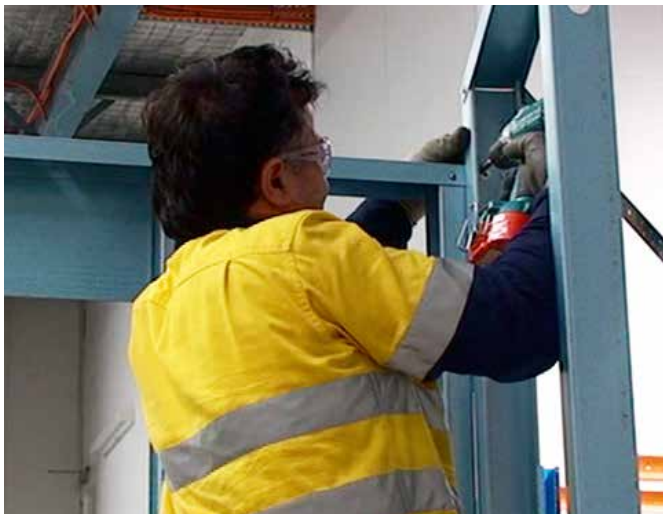
Figure 7.25 Once the frame is plumb and square, fix at the top of the wall.
