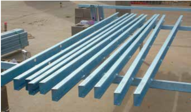
Figure 6.19 Layout all studs in sequential order, space out & orientate frame as per assembly sheet.
