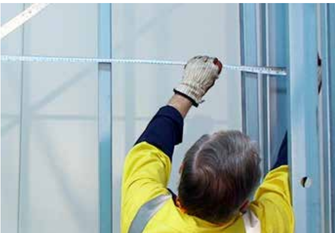
Figure 7.22 Measure lengths at bottom and top of wall to check frame is square.
