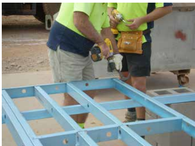
Figure 6.27 Fix bottom plate to studs, align holes & screw fix all noggings & bottom plate connections on "Side A". (Easier to fix bottom plate on an angle, starting at one end & pinching studs into plate, working along the frame). Ensure ENDUROTIE™ bent tab stud alignment is correct.
