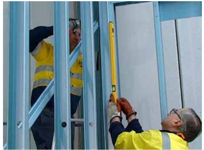
Figure 7.26 Use a length of TOPSPAN batten to hold the frame square until bracing can be tensioned.
