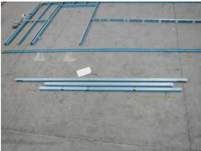
Figure 6.13 Separate and move stud & nogging / plate frame packs next to designated assembly zone.
