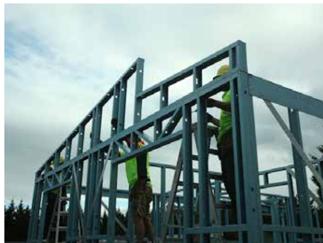
Figure 7.14 End wall placed into position and temporarily braced using clamps and/or TOPSPAN battens.
