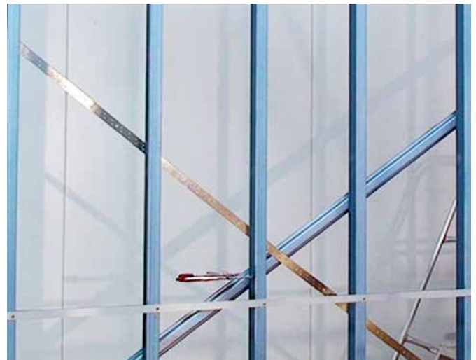
Figure 7.27 Use strap bracing and tensioner to set frame square and plumb. Note vice grips at mid-span.
