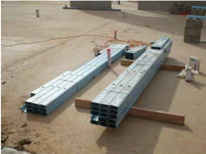
Figure 6.12 Locate & open matching stud & nogging / plate bundles before separating into individual frame packs.
