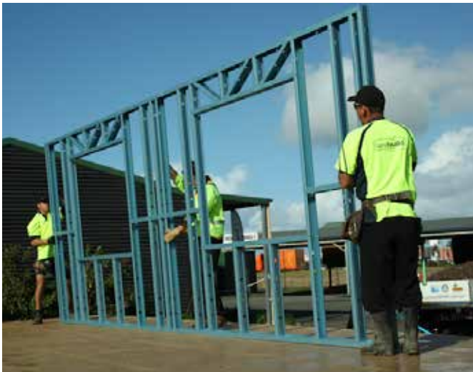
Figure 6.31 Ensure sufficient labour available on both sides of frame to flip safely.
