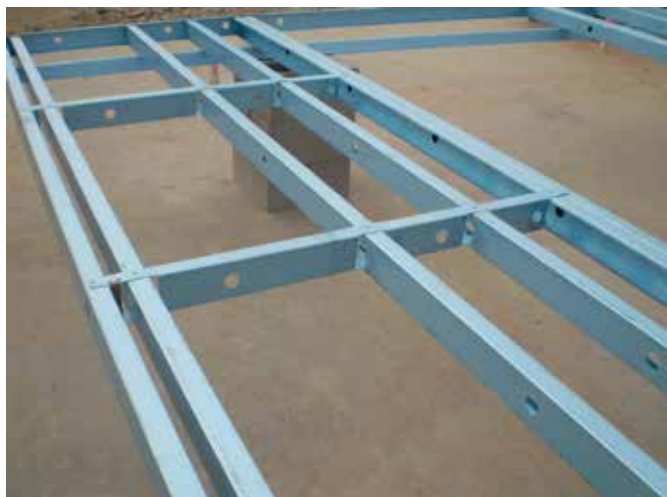
Figure 6.25 Slide noggings onto the studs from base of frame & align fixing holes. May require 2 people to slide up studs evenly.
