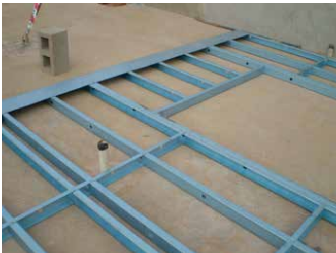
Figure 6.40 Completed wall frames to be stacked in a flat area ready for installation.
