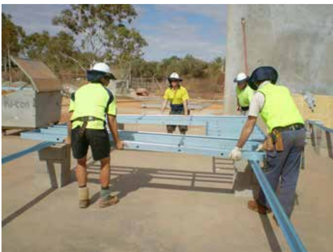
Figure 6.32 By utilizing two adjoining assembly tables, wall fabrication can be optimized by preparing the next frame while screw fixing & checking “Side B”.
