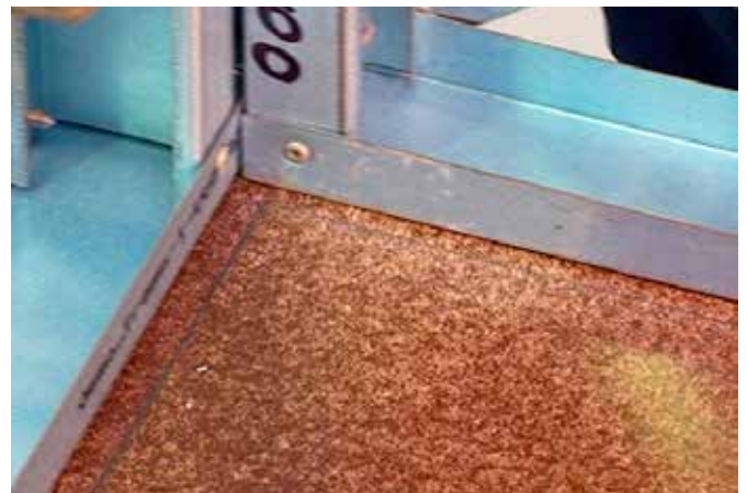
Figure 7.19 Align walls with chalk marks and put into final position before fixing.
